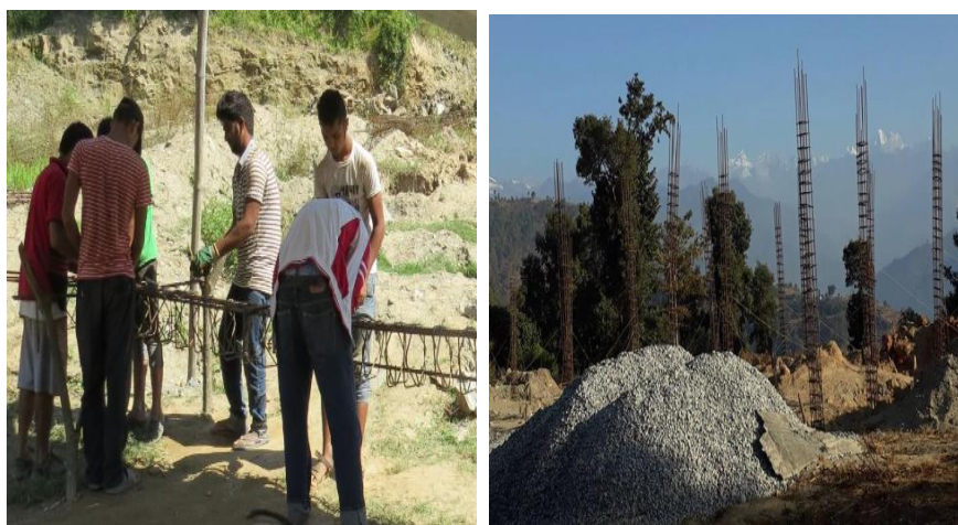
FIGURE 4. Youths engaged in work to prepare iron pillars (left) and pillars ready for concrete (right)
